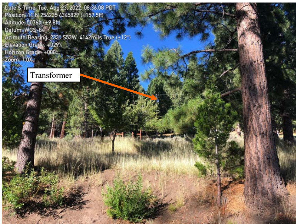
Looking southwest toward the pole-mounted electric transformer that serves the main residence.
