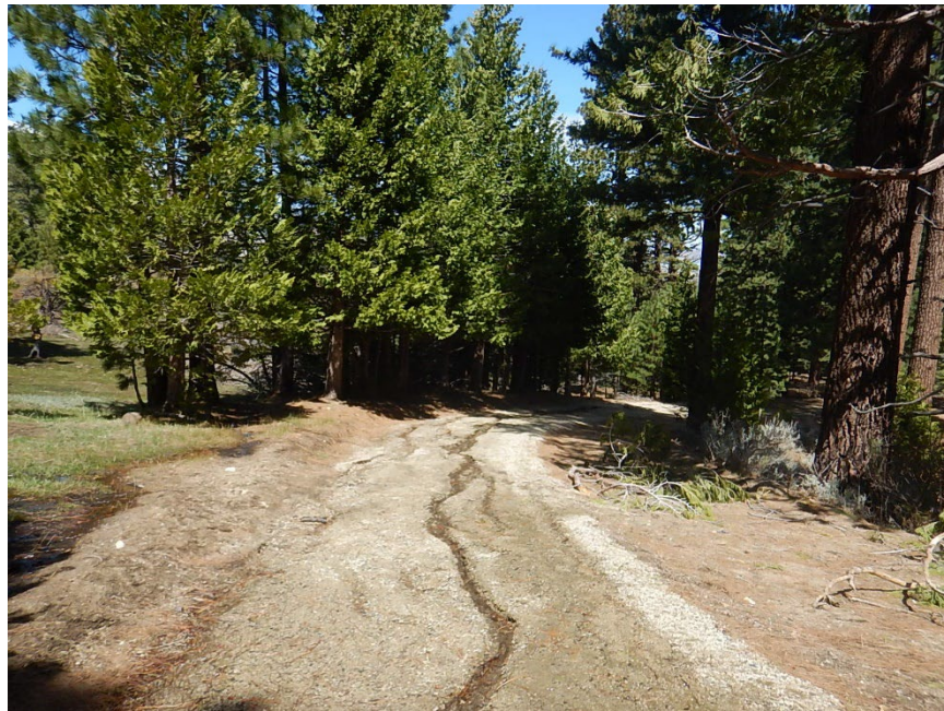
VIEW FACING NORTHERLY ALONG A GRADED ROAD WHICH PROVIDES ACCESS TO THE EAST PORTION OF THE SUBJECT PROPERTY
