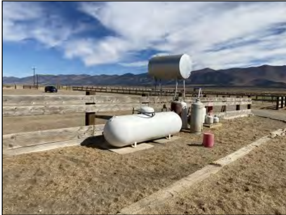
5 : View of the northeastern portion of the Subject Property - container storage including AST and propane.
