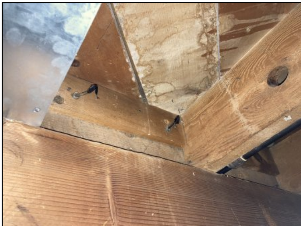
12 : View of cut copper lines suspected to be related to former heating oil furnace.
