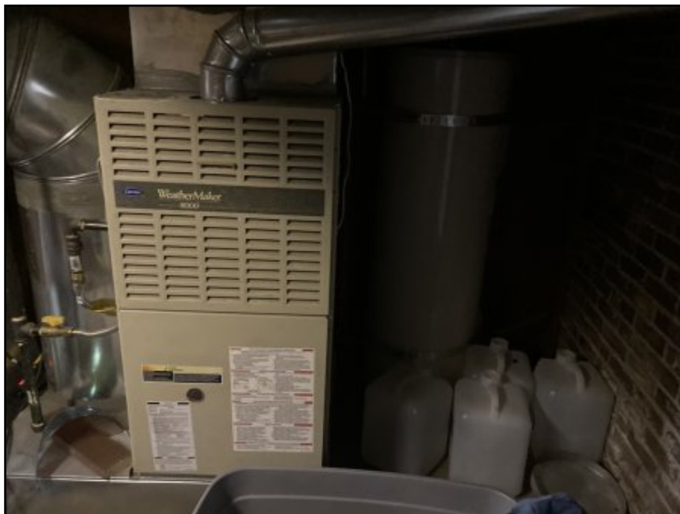
11 : View of the Subject Property furnace.
