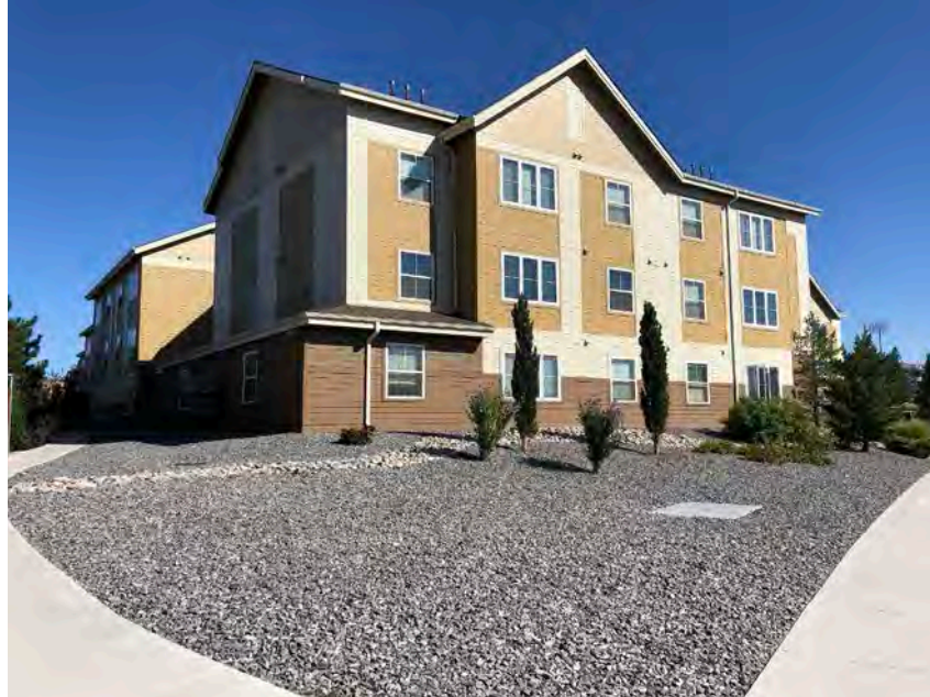
VIEW OF THE SUBJECT PROPERTY FACING NORTHEAST FROM EVANS AVENUE, NEAR THE SUBJECT'S NORTHEAST PROPERTY CORNER
