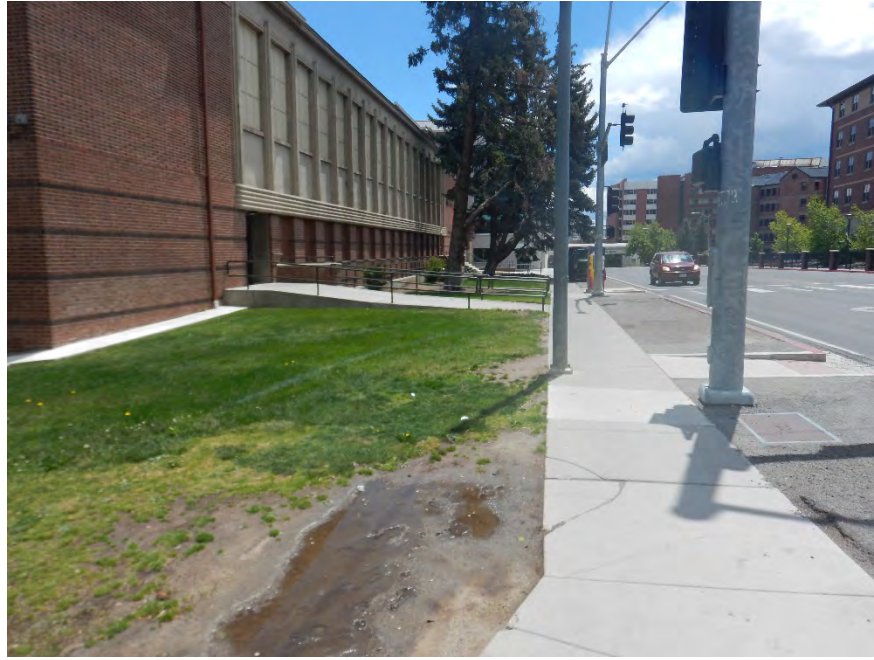
VIEW OF TEMPORARY CONSTRUCTION EASEMENT TCE-3 FACING SOUTHERLY ALONG NORTH VIRGINIA STREET AT COLLEGE DRIVE
