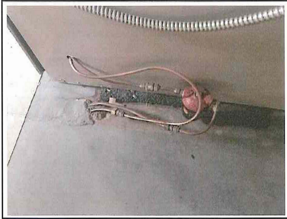
Photograph 9: View of the heating oil furnace located in the basement of the Subject Property.
